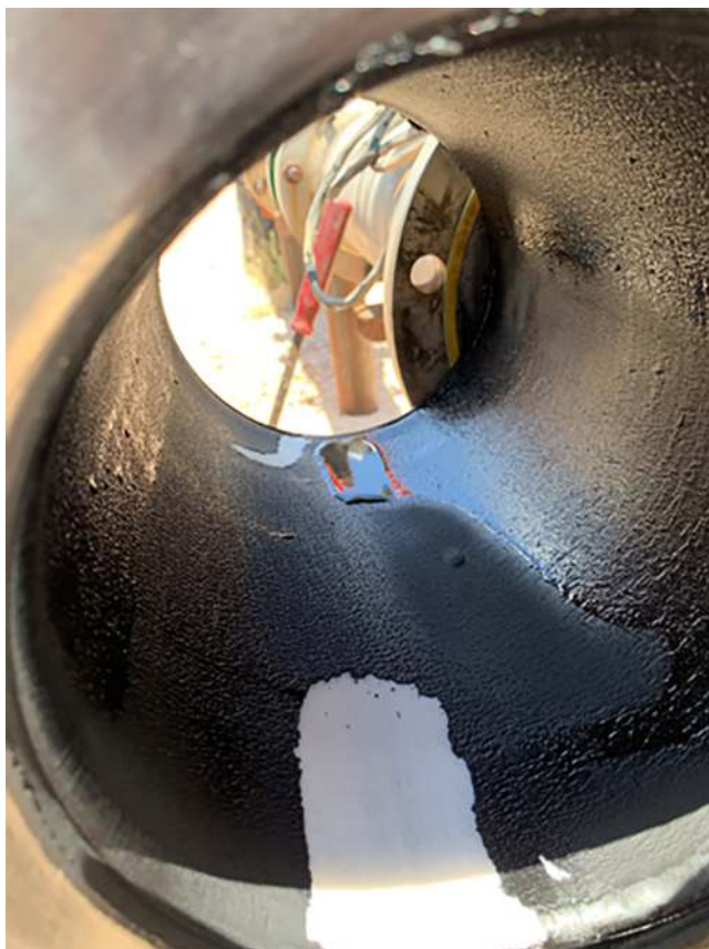
Fig. 1—Electromagnetic flowmeter fouled with paraffin prior to AMI treatment.
